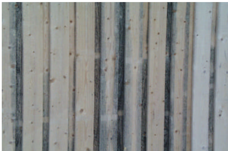
Figure 8. Mould and bluestain on wooden facade. Mould attack is varied on the surface.
